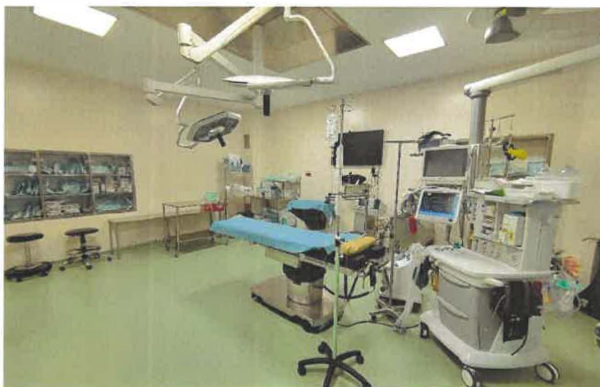
Automatizare bloc operator parter Casa Austria
